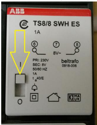
Image 15 – Turn on doorbell transformer
